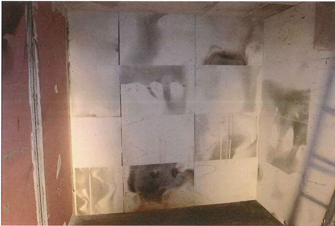
Figure 2. Calcium silicate board installed on the ceiling, rear wall and RHS walls. The LHS wall shows the fire rated plaster board substrate
