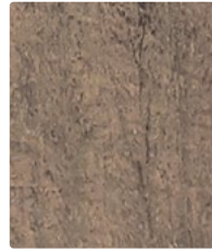
Oxidised Beamwood N C
